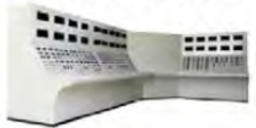
| Central Control Station
