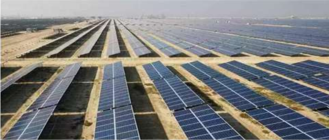
300MW utility PV plant in Bahawalpur Punjab
