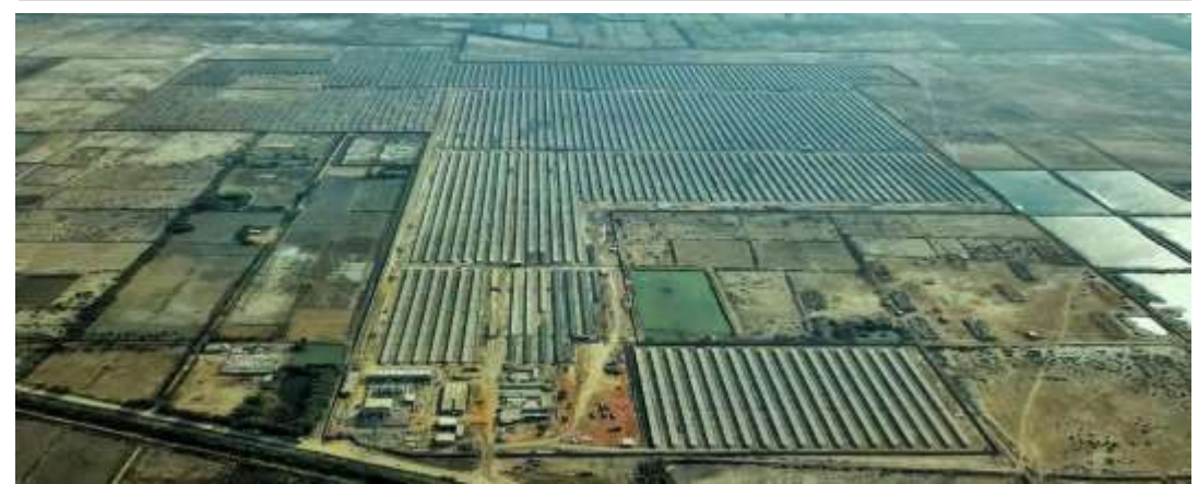
50MW Gharao Solar PV plant in Thatta, Sindh
