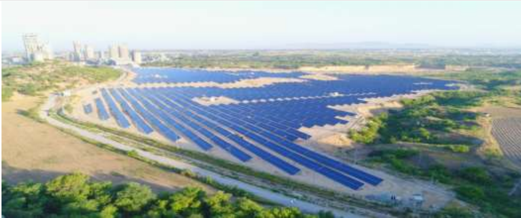
17.5MW PV plant of Fauji cement punjab
